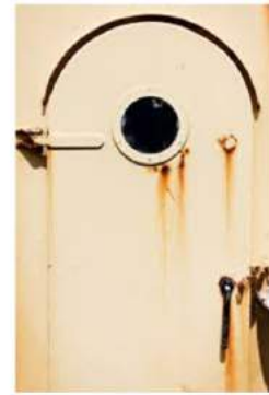
Fig. 15 Rust runner on door
