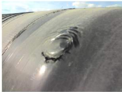
Due to Improper Curing
