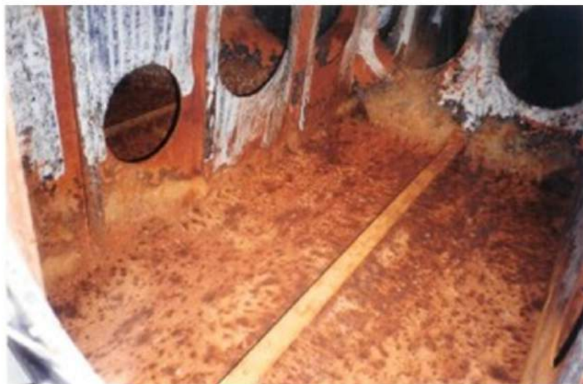
Fig.7 Corrosion in Ballast Tank
