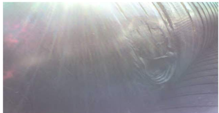
Fig. 12 Coating damage due to Fork Lift
